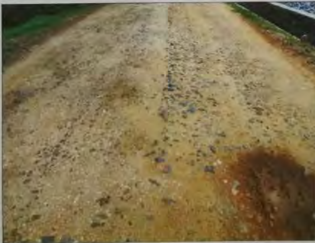
Fig. 64 A view of existing worn out surface at MGR road from Sirsoti to Ganyari Village
