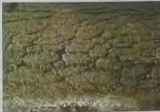
Fig. 75 Extensive alligator cracking on MP-1 road
