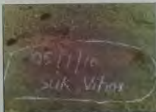
Fig. 45 Condition of repaired pot hole after two months at Sukhdev Vihar
