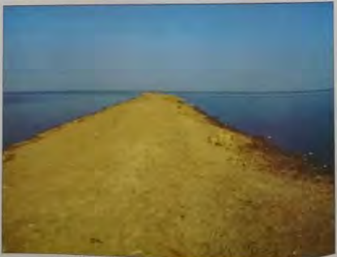
Fig. 29 A view of the border road to be constructed through water logged area
