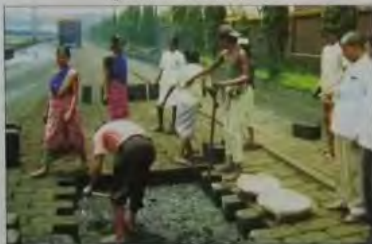
Fig. 31 Repair of failed section of in-use two lane road by concrete blocks
