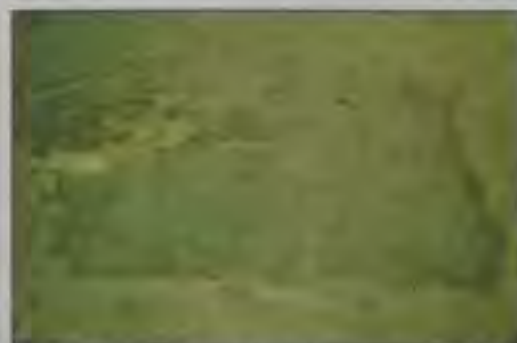
Fig. 78 Patching, potholes and loss of materials on Udyog marg
