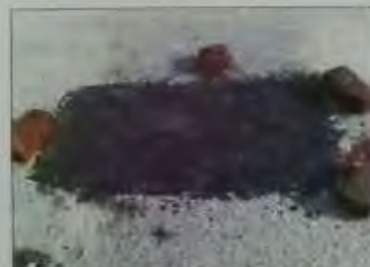
Fig. 44 A typical view of finished pot hole after its repair at Sukhdev Vihar road
