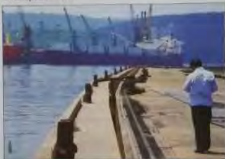
Fig. 30 Failed berth on the sea side
