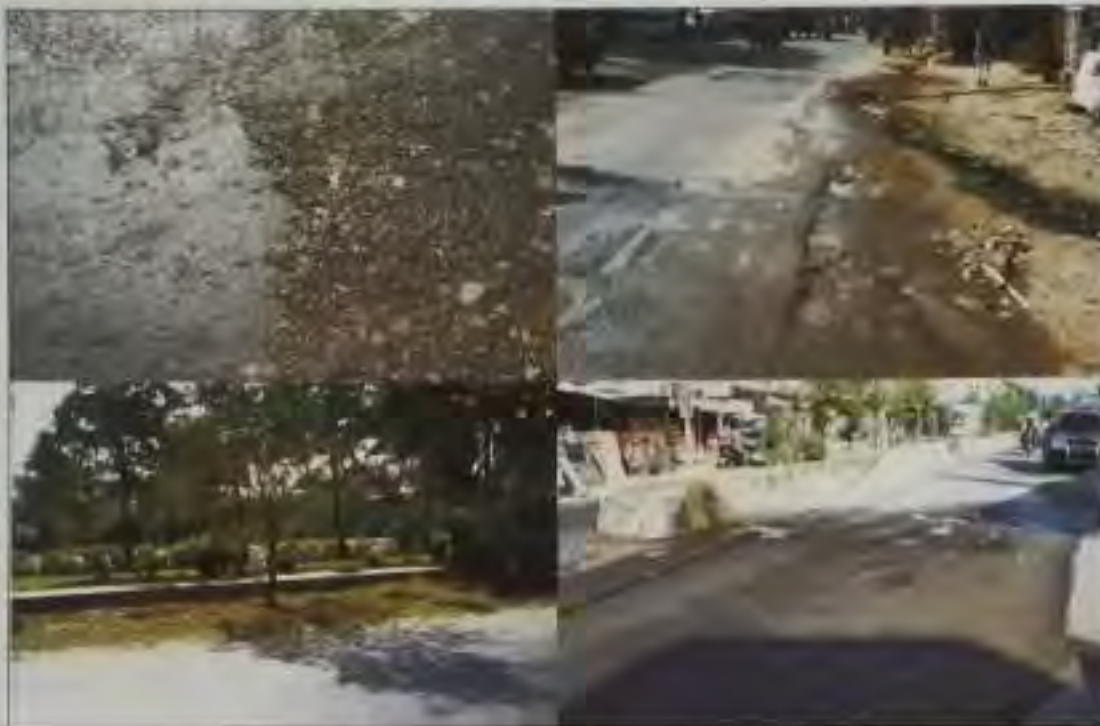
Fig. 41 Existing condition of pavement at the DSC road from Kulesra to Surajpur
