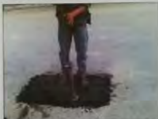
Fig. 43 A view of pot hole repair process (Compaction with Conventional Rammer) at Sukhdev Vihar road
