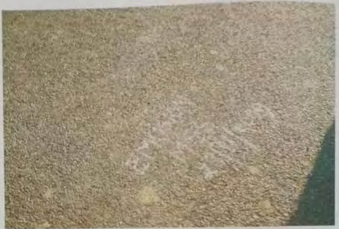
Fig. 34 Satisfactory performance of mix seal surfacing with emulsion on Dantaur- Khajuwala road after 2 years
