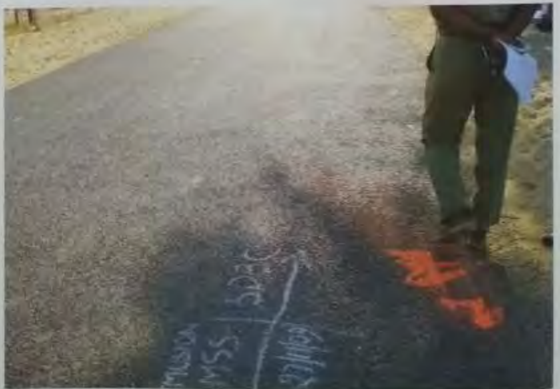
Fig. 35 Satisfactory performance of SDBC with emulsion on Dantaur- Khajuwala road after 2 years
