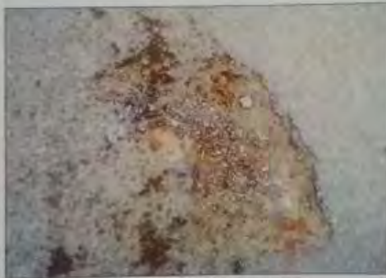
Fig. 37 A close up view of distressed surface
