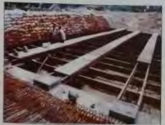
Fig. 93 Load testing of formwork of concrete girder at a bridge construction site on Gurgaon Feeder Canal
