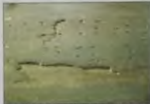
Fig. 76 Slippage at the intersection on MP-1 road
