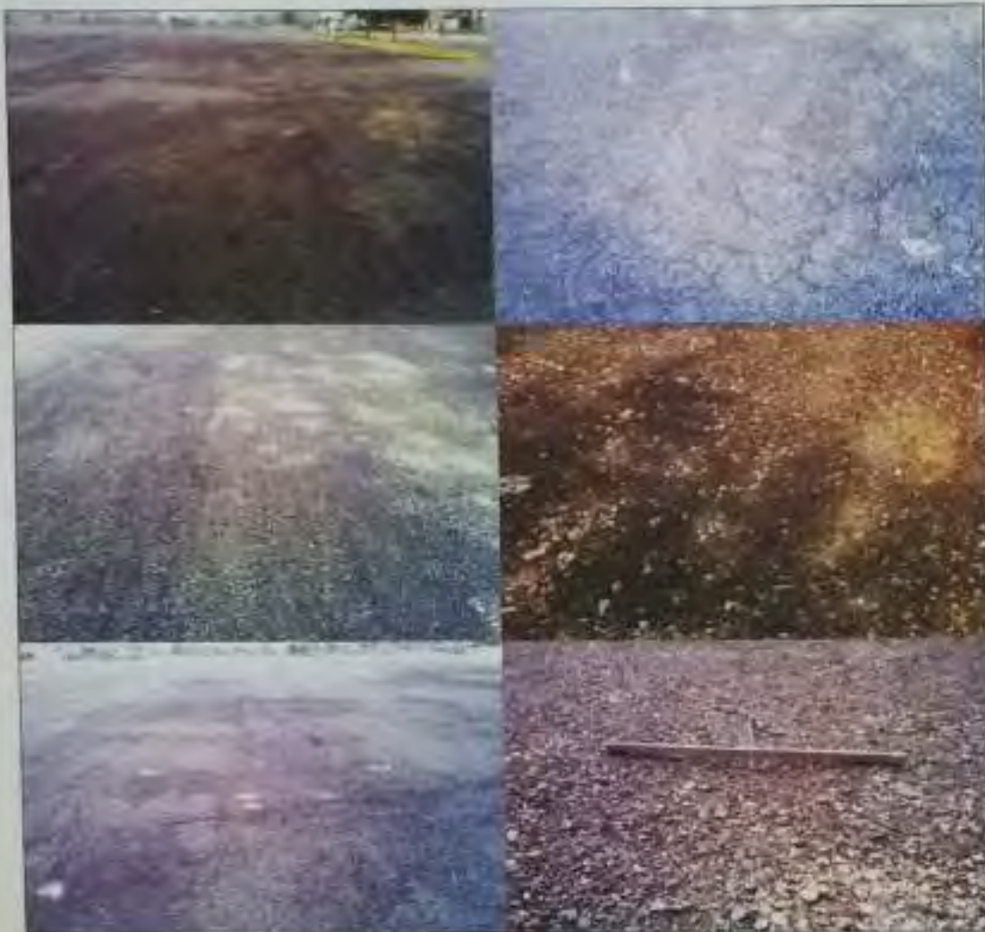
Fig. 40 A view of existing condition of pavement at the parking bay of IMT (Sector 3), Manesar
