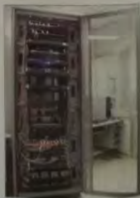
Fig. 147 Newly installed central switch & Firewall system
