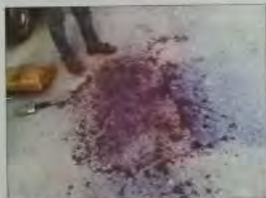
Fig. 42 Preparation of pot hole area in rectangular shape at Sukhdev Vihar road
