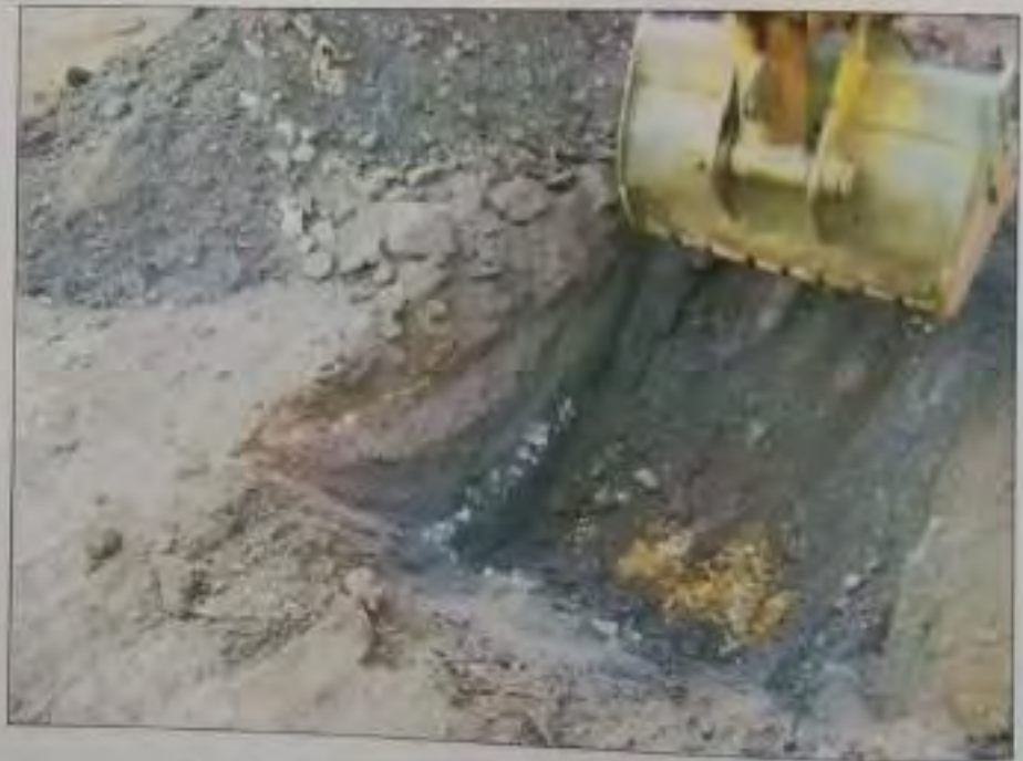
Fig. 33 Iron ore material on the surface H6 to SBC Road at DHC
