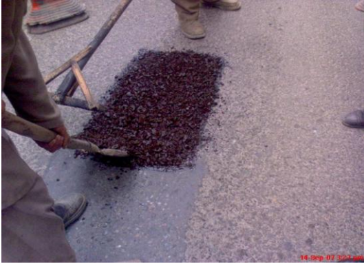
Patch work with cold mix in progress on NH-1A in snow and cold climate area in September, 2007 under Border Roads
