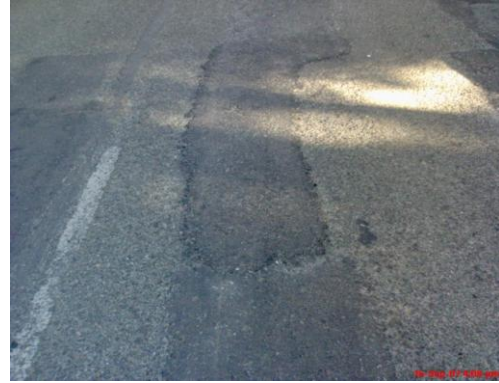
Intact Patch work with cold mix after week on NH-1A in snow and cold climate in September, 2007 under Border Roads
