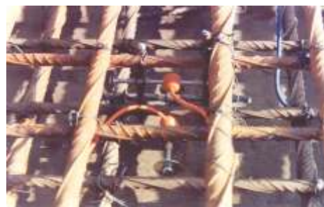
Installation of V W Strain gauges at Lok Nayak Setu, New Delhi
