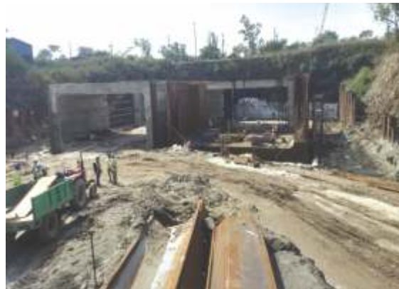
Construction of Rail Underpass by Box Jacking with Soil nailing at Pragati Maidan
