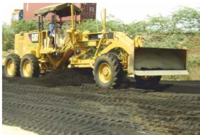
Stacking and spreading of copper slag by grader, Madurai-Tuticorin expressway, Tamil Nadu
