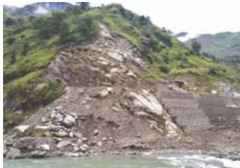
Investigation, Design and Remedial Measures for protection of slopes at Bailey bridge, Pambai Valley
